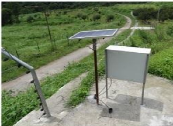
Solar Panel and control Unit
